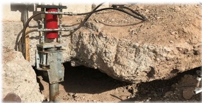
Typical pile with lifting jack. The gap under the footing shows how much was lifted
