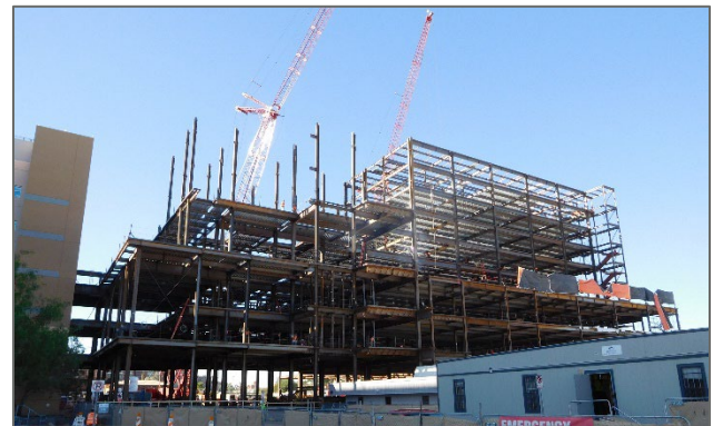
Steel framing (erected by two large cranes) started after foundation was complete. Slab on grades were not poured until after steel was erected.
