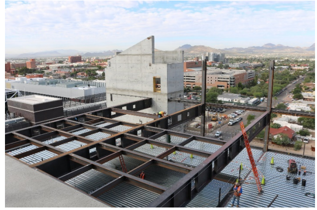
Typical floor framing with 90' steel plate girders. Holes in steel girders for MEP ducts and piping
