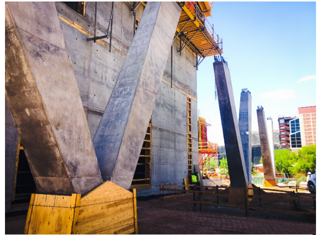
Two story ‘V’ columns looking north- special concrete forms used to frame the concrete
